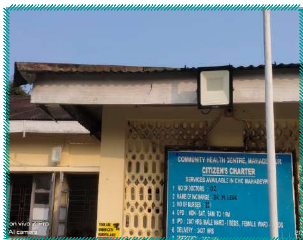
Outdoor Light installed at CHC Mahadevpur
