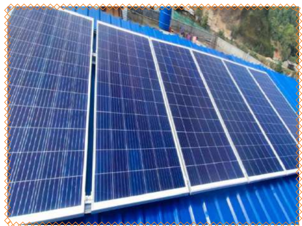
Solar panels installed at roof top of CHC Pakke Kessang
